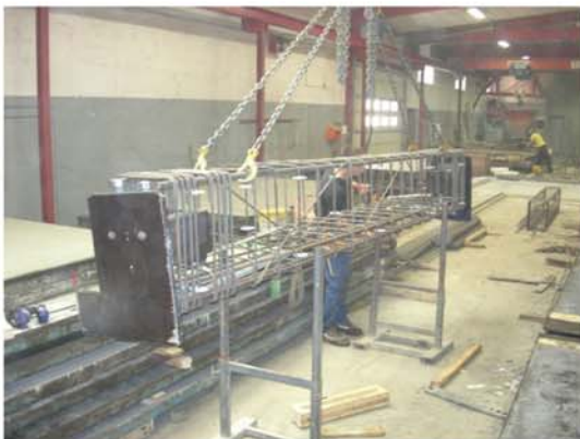
P17. Completed reinforcement with the BCC unit inside, is lifted to the casting mould.
